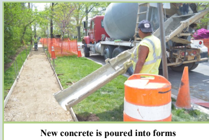
New concrete is poured into forms
